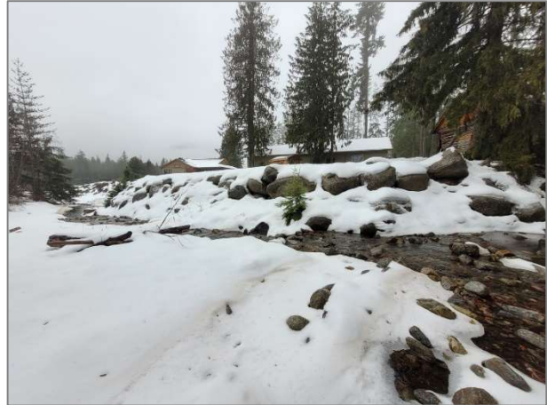
Photo 10. View of right bank and lower fencing location, with riprap along bank.
