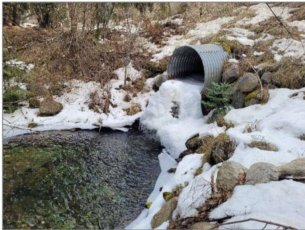
Photo 7. Perched culvert outlet under Hwy 3A.
